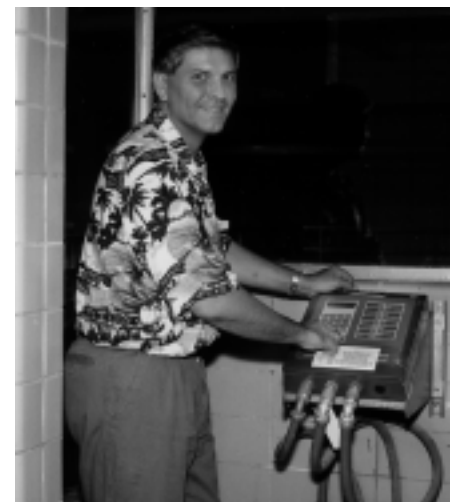
David Milcinovic, Water Plant Operator 1, uses a Pakscan IIS unit to control Rotork operated valves in the filtration building.
