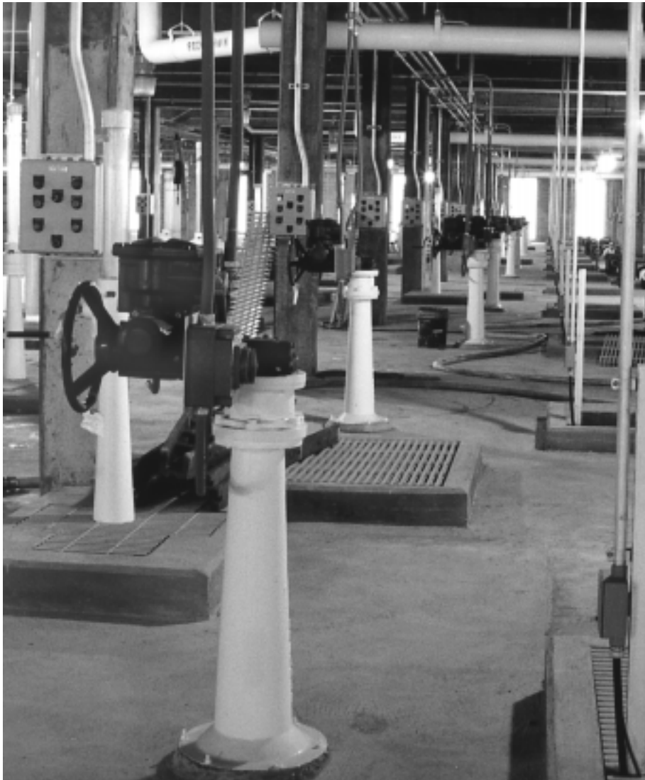
Rotork IQ actuators work every two minutes, 24 hours a day in order to maintain the appropriate water level above Crown's filters.
