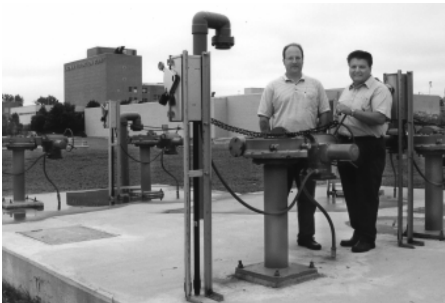
Richard Papp, Plant Manager, (at left) and Nevio Bais of Northcoast Process Controls, Inc. discuss aspects of the renovation project. Northcoast Process Controls worked closely with Crown personnel to install and commission the Rotork actuators and Pakscan system.
